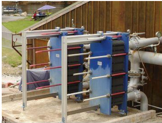
Figure 2.6. Plate heat exchanger at the Taupo Prawn farm (Thain et al 2006)
