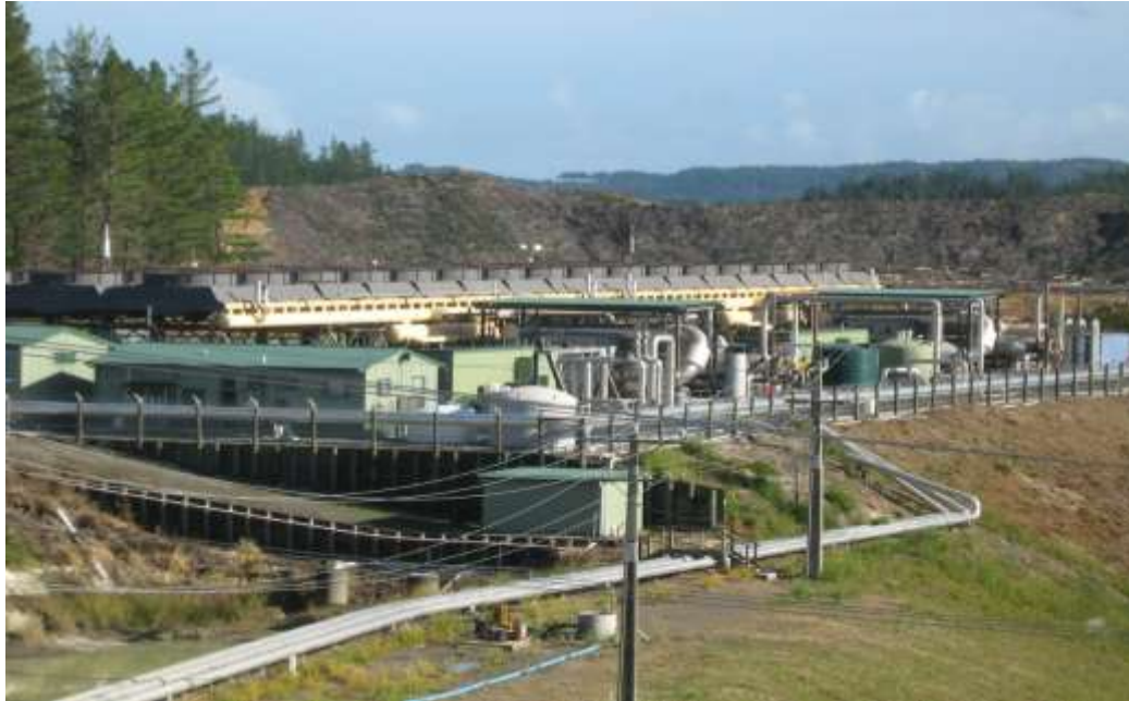
Figure: Station 1, 10MWe Ormat binary plant commissioned in 1998
