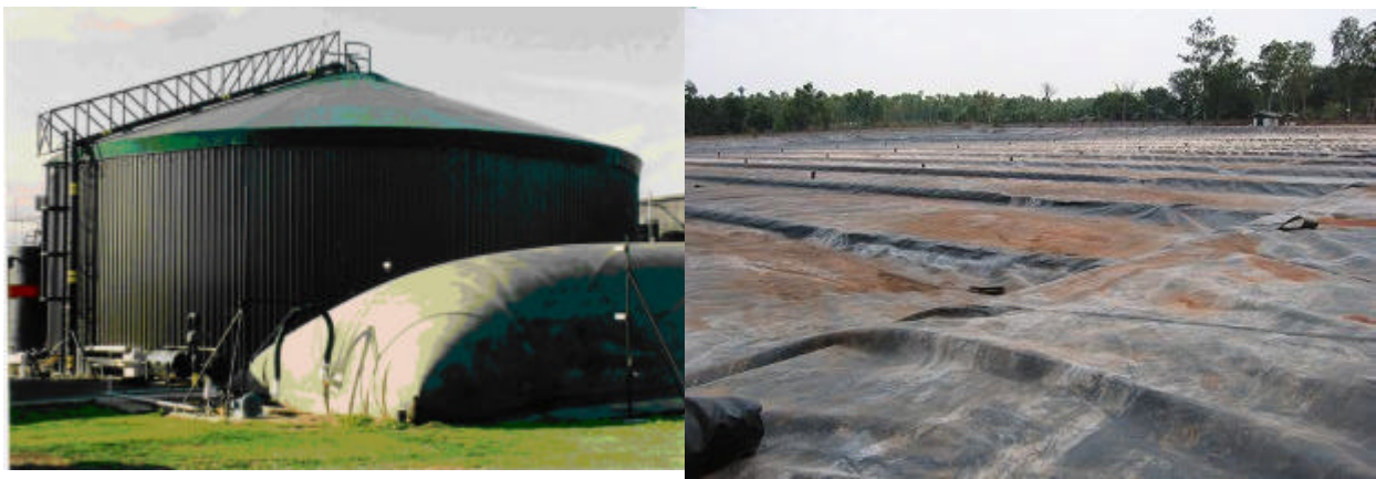
Figure 1 (Left). WSL completely mixed digester for food residuals and high fat waste.
